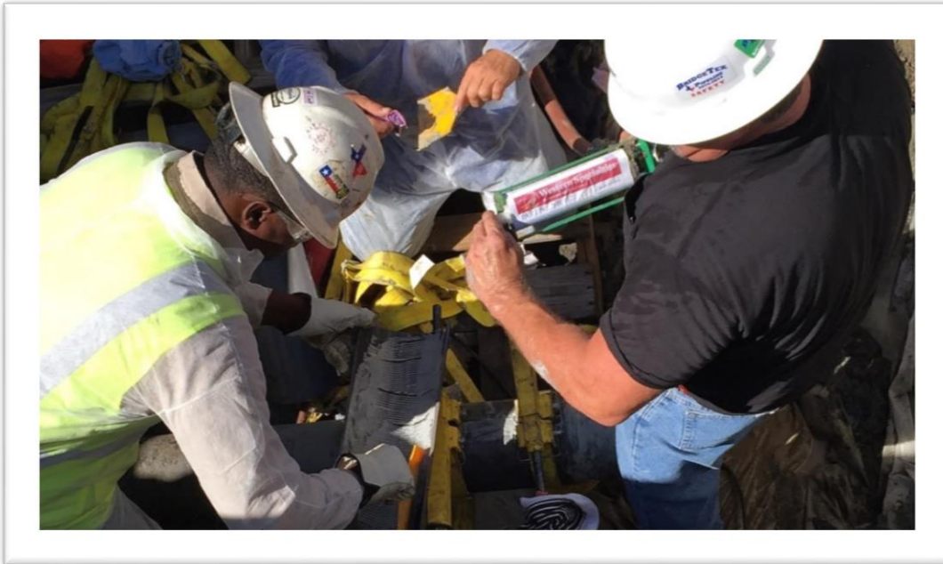
Application of patented adhesive to both the steel sleeves and pipe surface.
