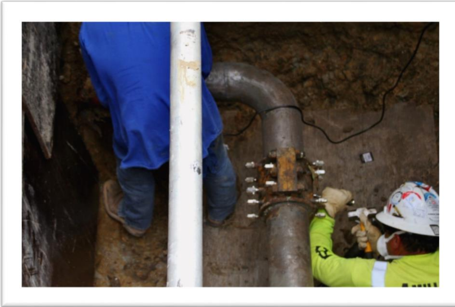
Leak clamp removal of Excavation B. While looking for good coating to determine the re-coat area, once the sleeve is installed.
